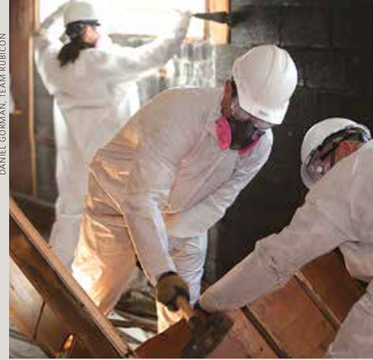
Operation: Greased Lightning Rockaway Peninsula, New York Superstorm Sandy 2012
