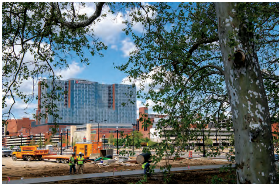
Construction projects such as Ohio State's Cannon Drive relocation are designed to mitigate the flooding dangers posed by climate change.
